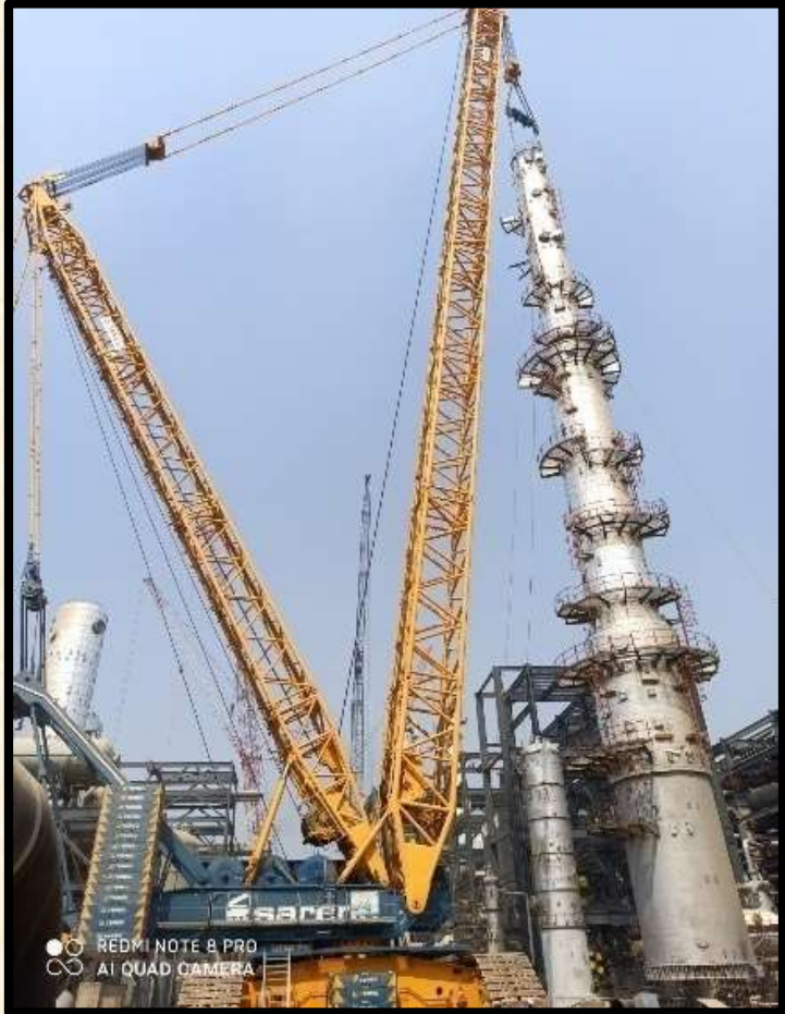
Erection of 1370 MT Equipment by 3200 MT crane and 1600 MT trailing crane at Bathinda Refinery of HPCL-Mittal Energy Ltd.
