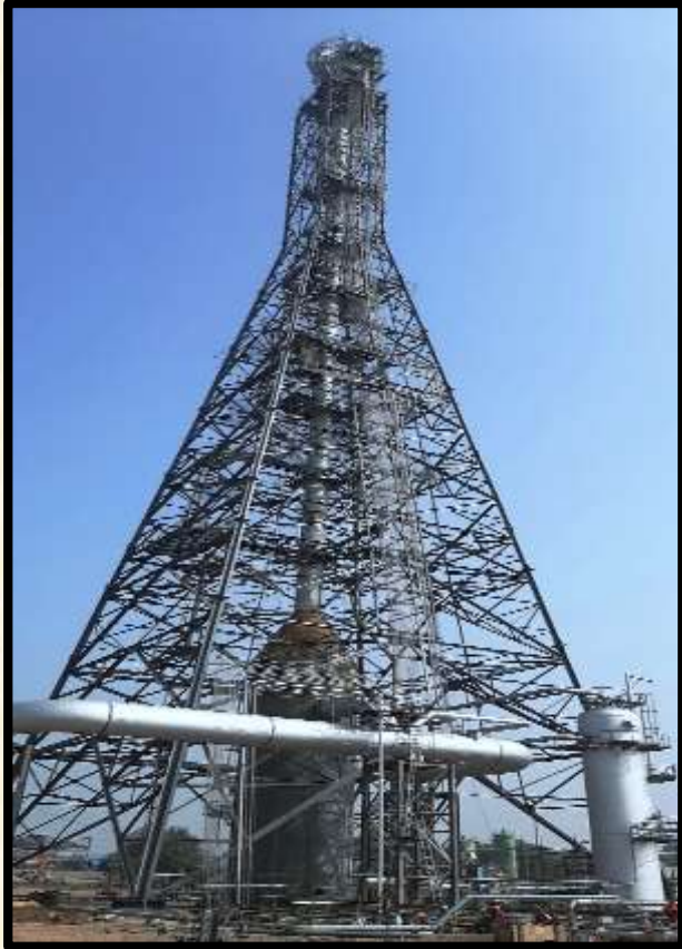
Flare Stack Structure - 135 Mtr. height at BS VI at Gujarat Refinery_vadodara
