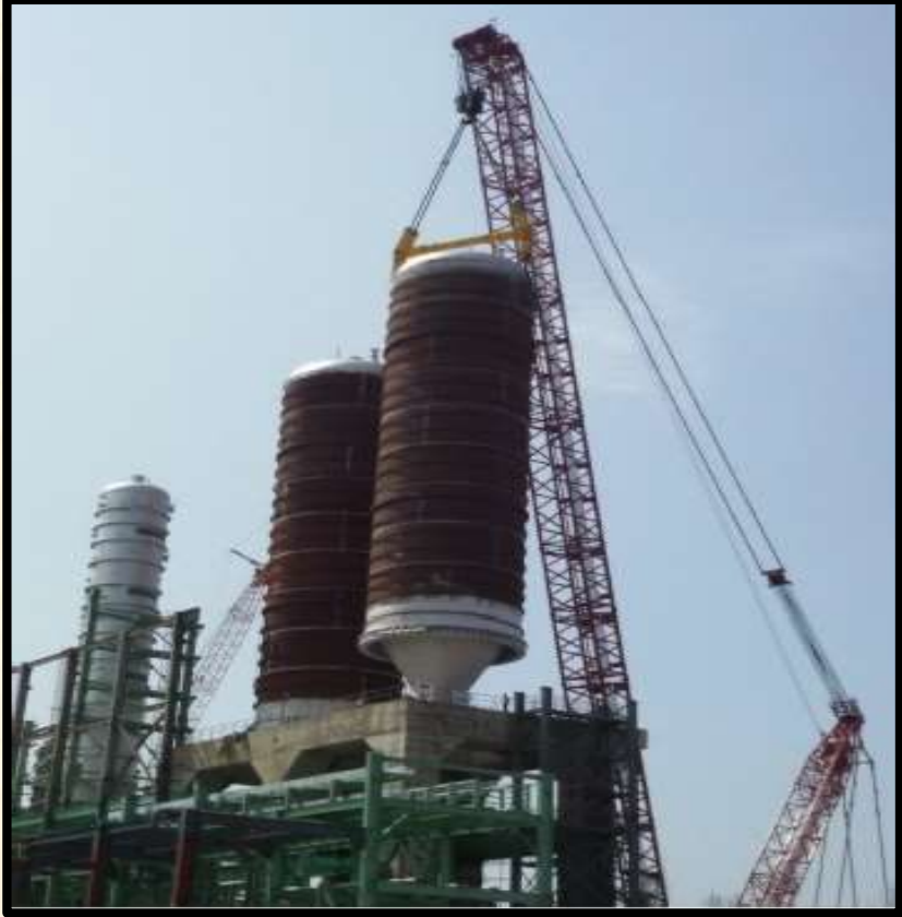
Erection of Two Coke Drums of 575 MT at DCU, Chennai Petroleum Corpn. Ltd. by Main crane 1250 MT capacity and tailing crane of 550 MT
