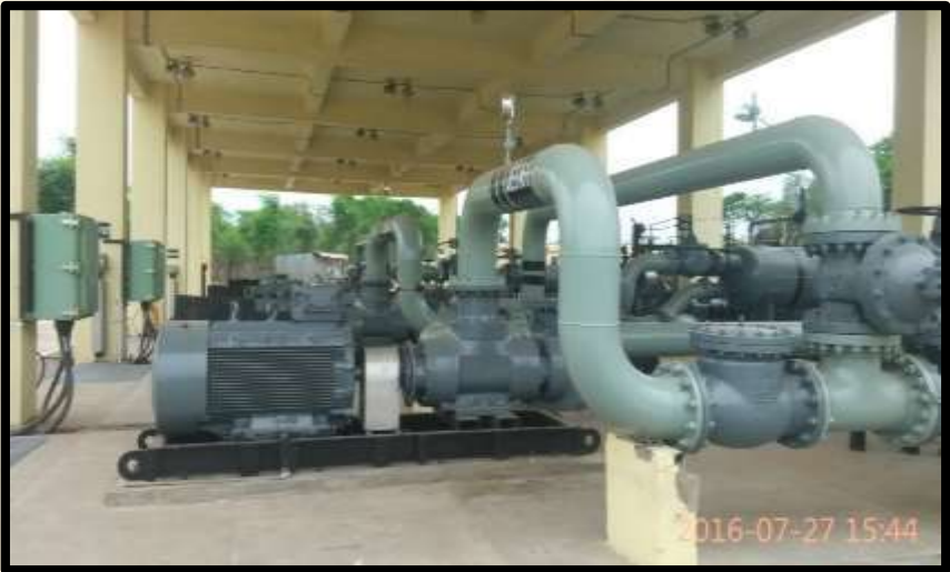
Hydrant Refueling Line at Hydrant Refueling Aviation Farm at IOCL Pune
