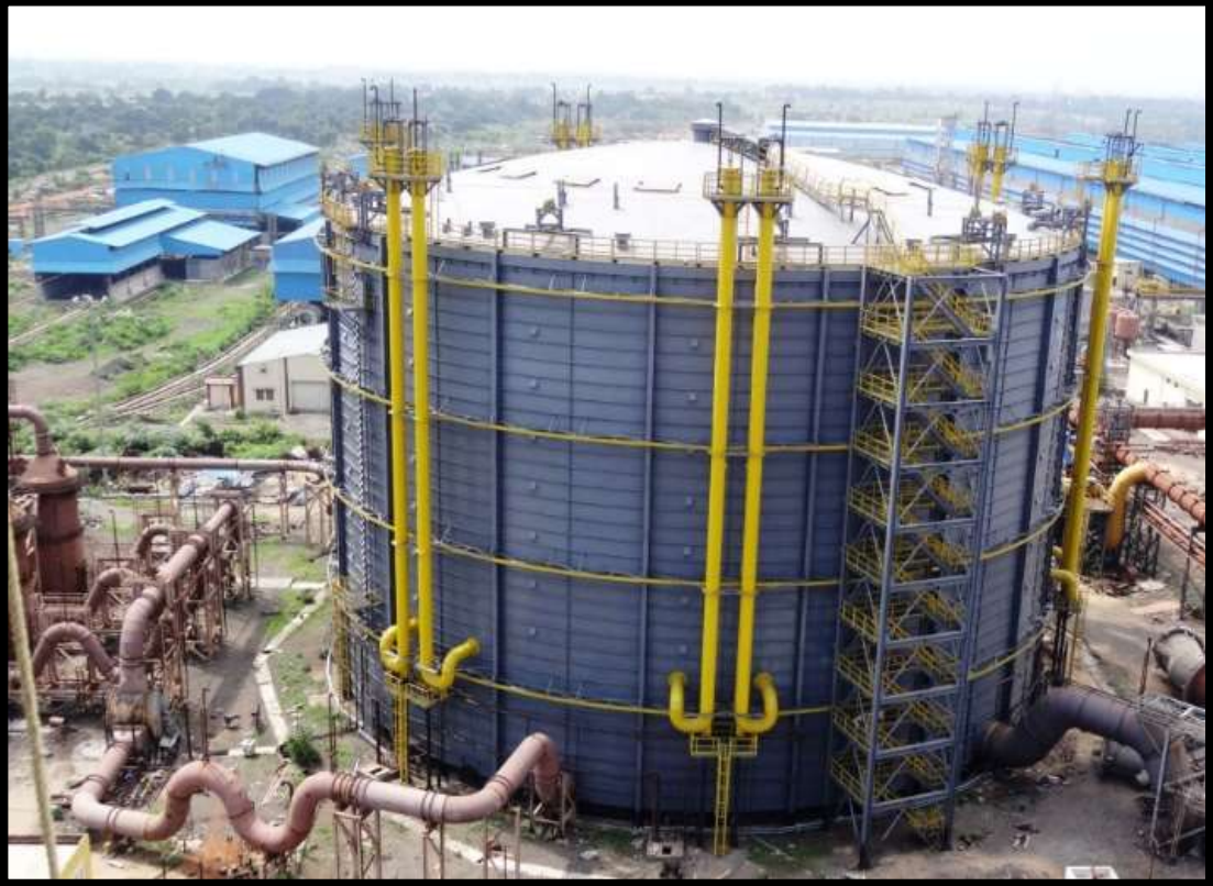
BOF Gas Holder for IISCO Steel Plant, Burnpur of Steel Authority of India Ltd.
