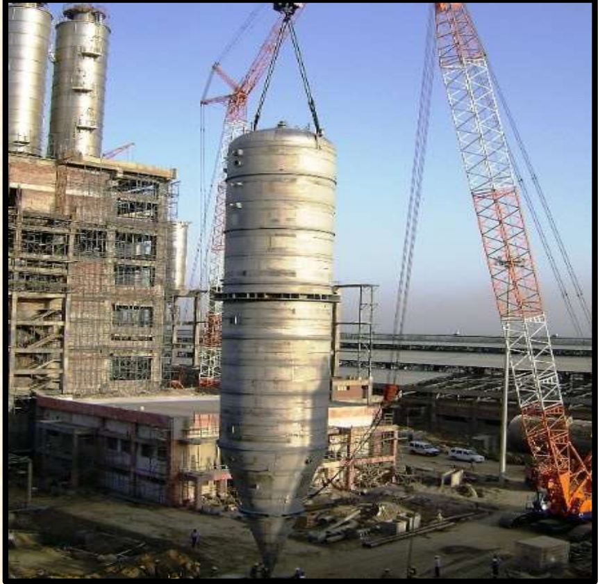
Mechanical Works for LLDPE-HDPE Unit for Panipat Naptha Cracker Project of IOCL
