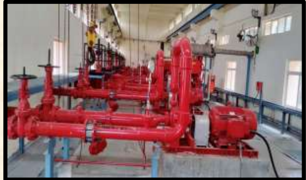
Performance Test For Fire Fighting System at BPCL Bina.
