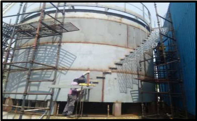
ATF Tank at Kolkata Airport for Reliance Industries Ltd.
