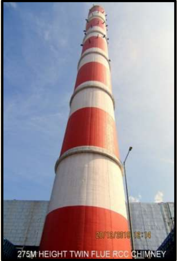
275M HEIGHT TWIN FLUE RCC CHIMNEY Construction of 275 M high RCC twin flue RCC Chimney at NTPC 2X800 MW STPP at Gadarwara
