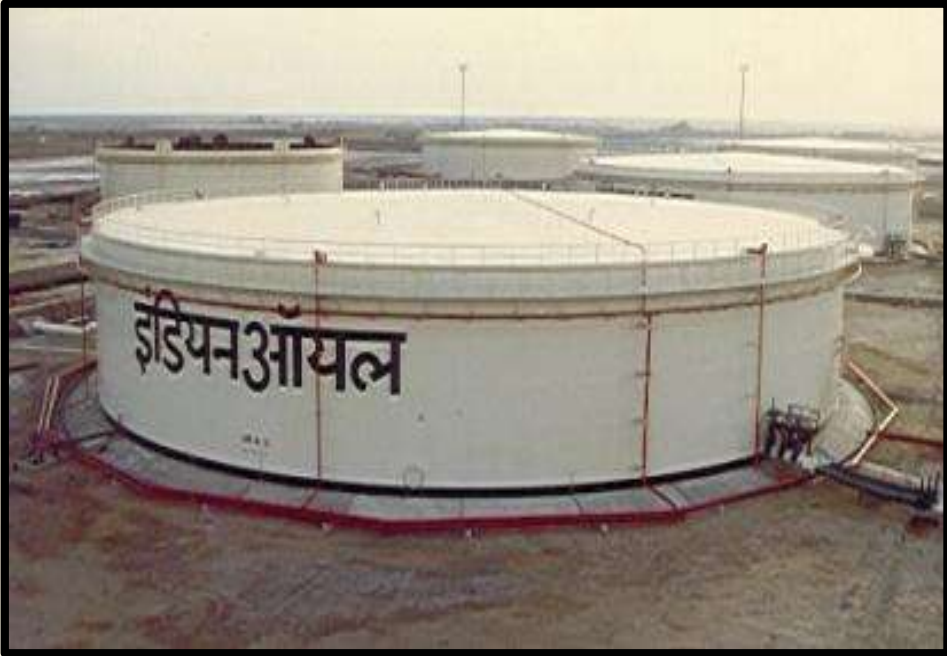
Product Storage Tanks with connecting pipeline at IOCL Kandla
