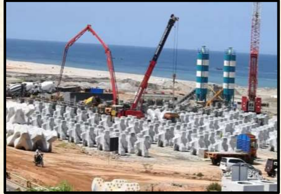
Casting and Staking of Accropodes for break water development of Vizhinjam Port at Kerala of Vizhinjam International Seaport Ltd. For Adani Group
