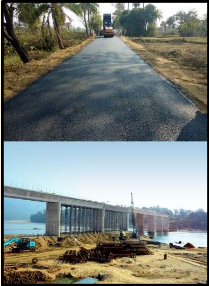
197 Km rural road connecting 74 villages in Malkangiri, Koraput & Sundargarh districts under PMGSY scheme in Odisha
