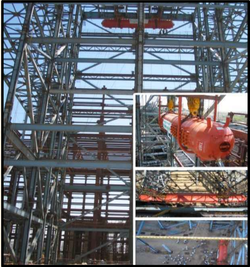
Erection, Testing & Commissioning of Boiler including Structures, Air Pre-Heater & Piping of 2x210 MW, Unit - 4 & 5, Bakreswar of Power Development Corpn. Ltd. for BHEL
