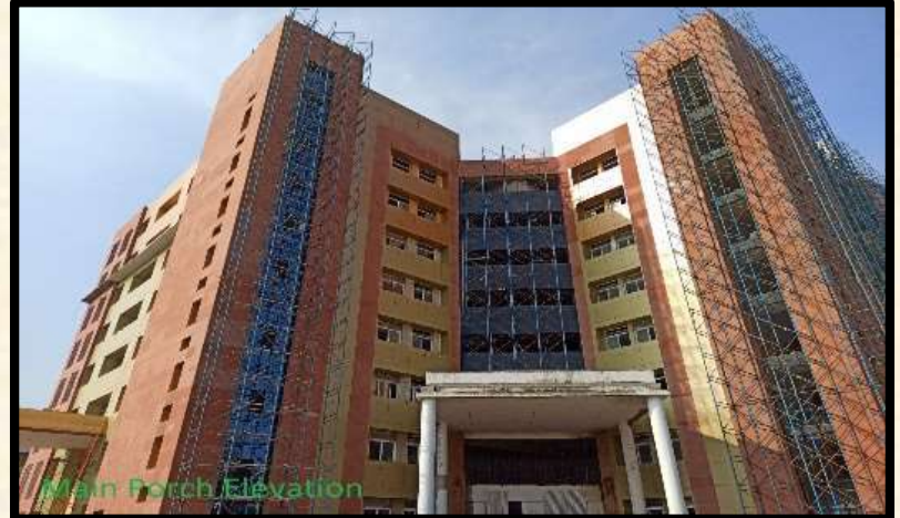
SMS Medical College,, Bhavnagar Construction of Super Specialty Hospital for Ministry of Health & Family Welfare under PMSSY Scheme
