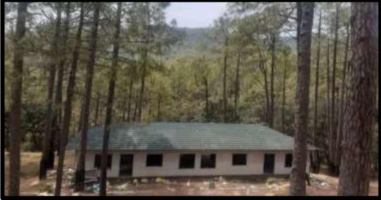
Construction of Eco Tourism destination at Titalikhet, Almora, Uttarakhand Forest Resource Management Project, Govt.of Uttarakhand
