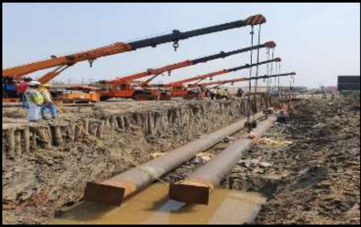
Propane and Butane pipeline Double Wall 18"/25" size Cross-Country Pipeline for BPCL Haldia
