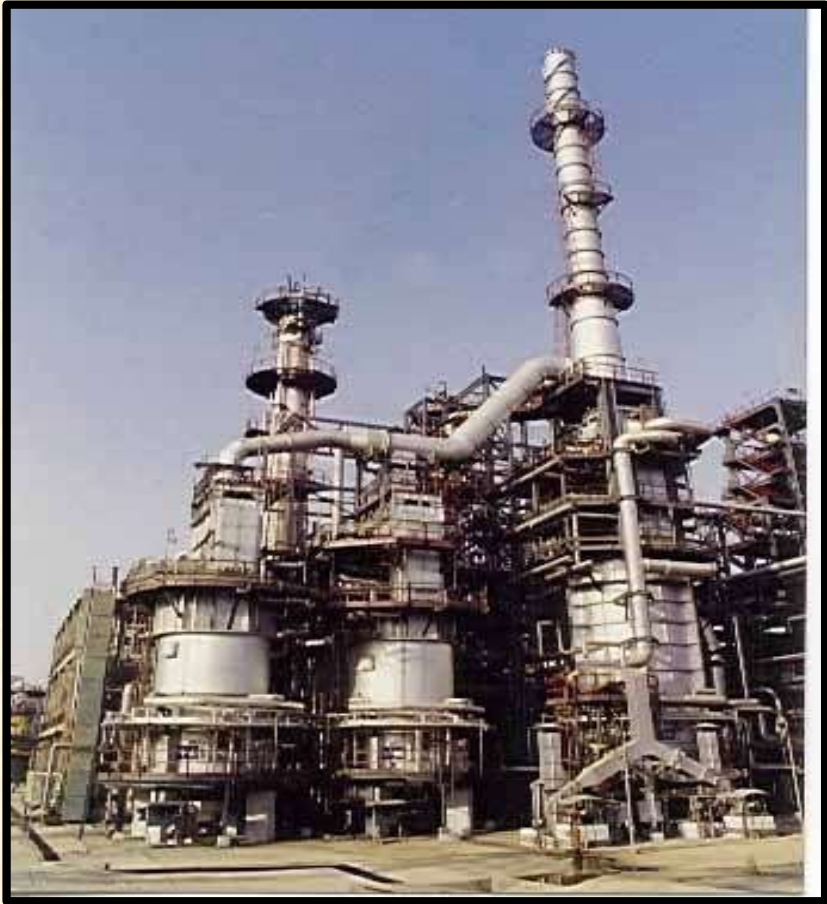
Turnkey Construction of 3 Nos. Non-IFP Heater in Panipat Refinery Project of IOCL, for Hydrotreater Reactor, Reboiler & Stabilizer Reboiler
