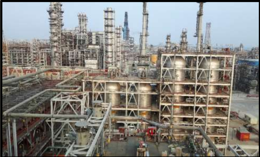
VGO-HDU Unit at IOCL Paradip Refinery
