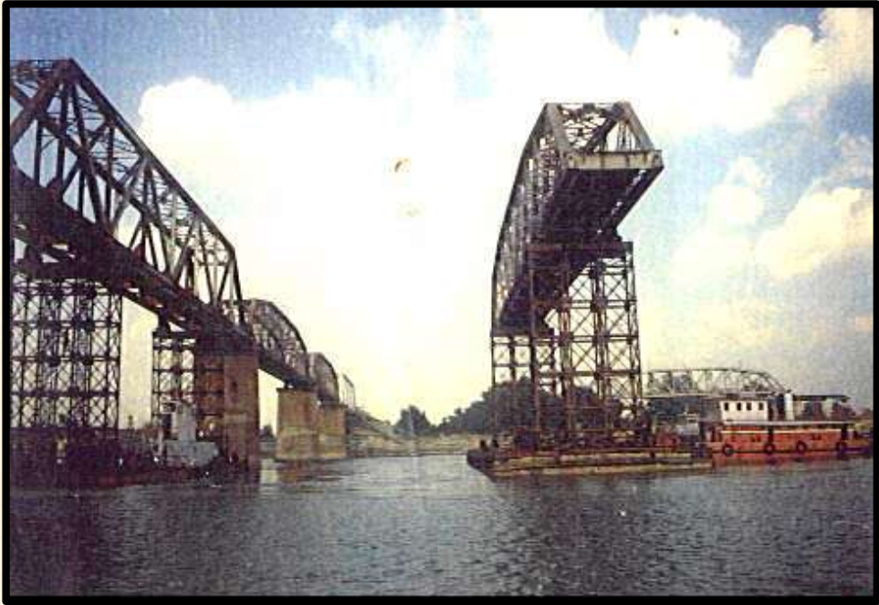
Regirdering of Railway Bridge at Majhi Ghat, Bihar for Northeast Frontier Railway
