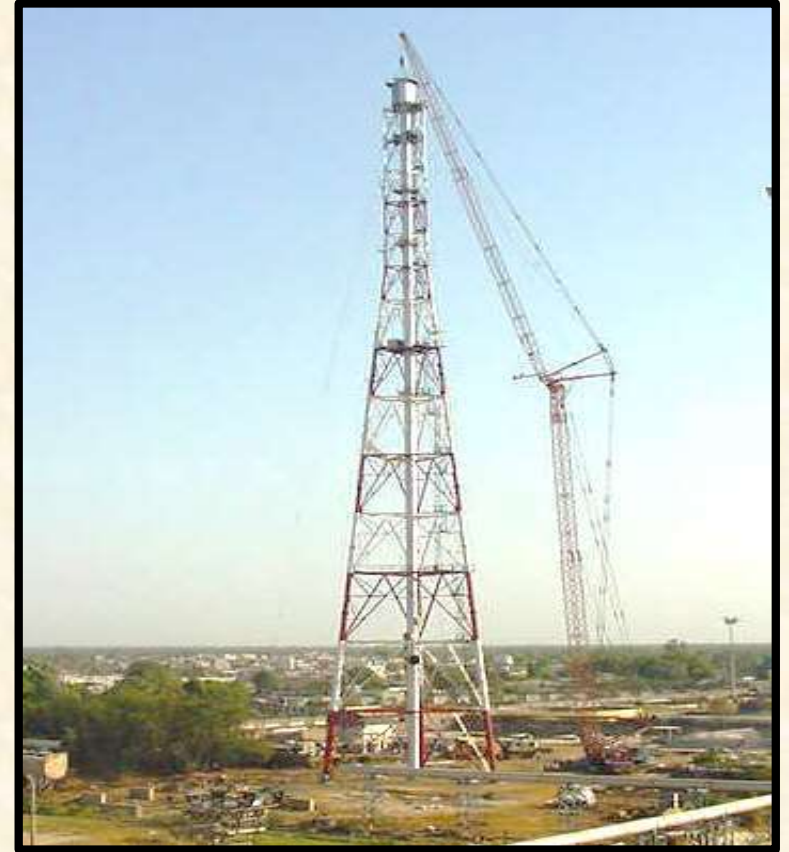
Erection of Flare Tip during Flare Stack Package on EPC Basis at IOCL Gujarat Refinery
