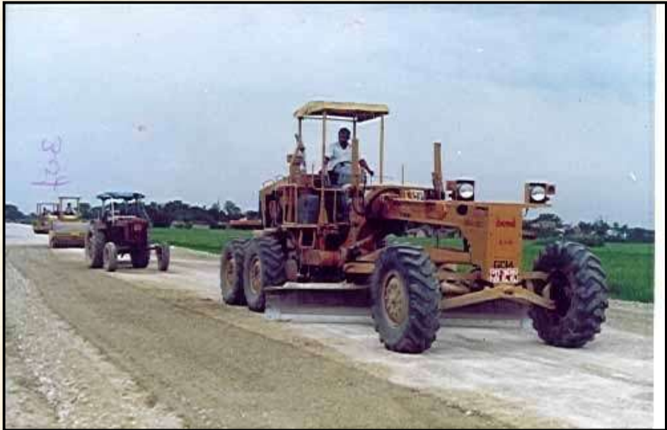
Construction of 2 lanes Durgapur Expressway with grade intersections & repairing of minor bridges & culverts, toll plaza & service road at Dankuni, W.B.) for National Highways Authority of India
