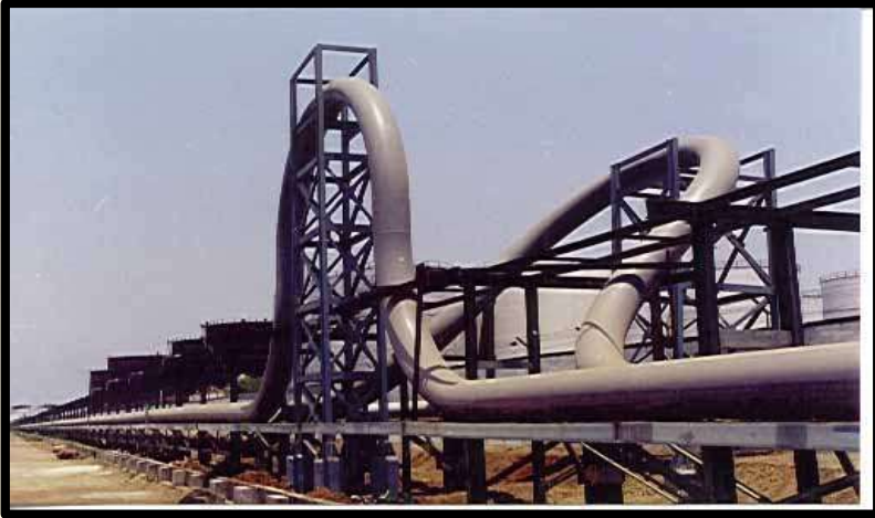
Cross-Country Pipeline for transportation of Black & White Oil for Oil Terminal of Indian Oiltanking Ltd.
