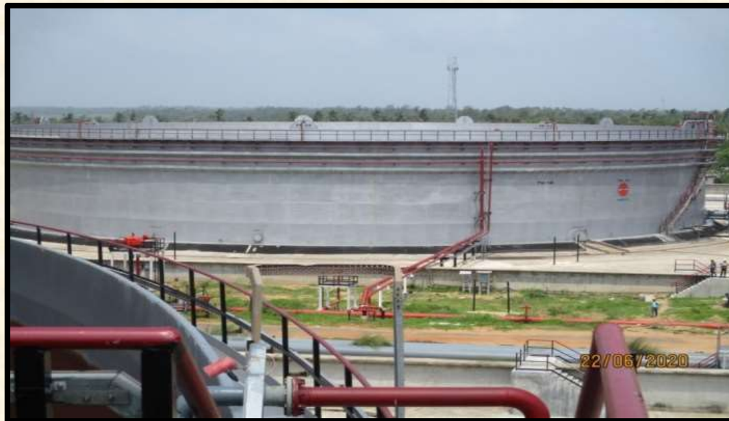
Turnkey Construction of 79 M Dia Double Deck Floating Roofs at IOCL Paradip Refinery
