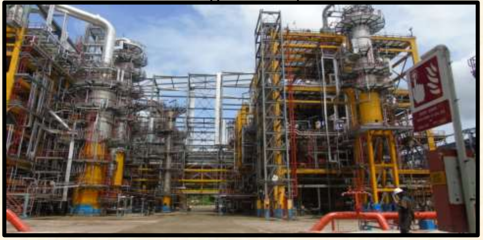
Acrylate Unit at BPCL Kochi Refinery
