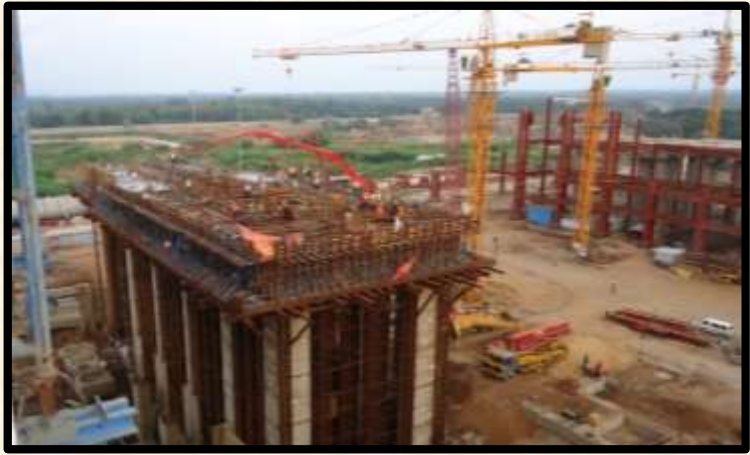
Balance of Turbine Island (BOTI) Package for 2 X 700 MW Kakrapar Atomic Power Project ( Unit 3 & 4) of Nuclear Corporation of India Ltd.
