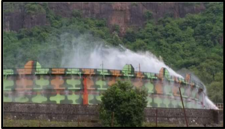
Fire fighting system for Crude Oil Storage Tanks at ONGC, Uran.
