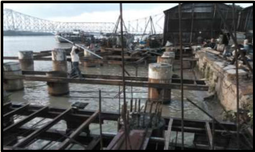
Construction of RCC Deck Slab supported on RCC MS lined Bored Pile of 1000mm dia., beam including pavement for Hooghly River Front Development Work of Kolkata Municipal Corporation
