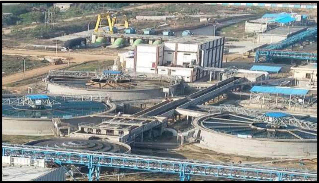
Water Pre Treatment and Liquid Effluent Treatment Plant at MUNPL Meja, Allahabad
