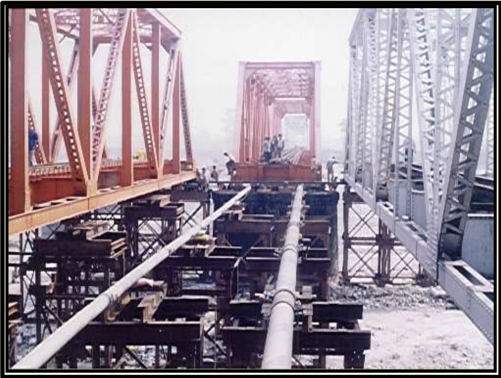
Regirdering of 7 spans X 45.70 metre each of Diana Bridge for Northeast Frontier Railway
