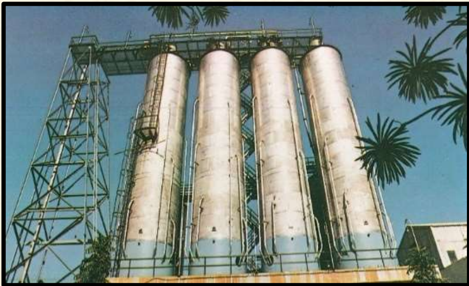
Stainless Steel Silos at IPCL Vadodara
