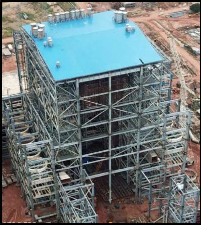
Boiler, Bunker & Allied Works for 2 X 800 MW Ramagundam STPP of NTPC Ltd.
