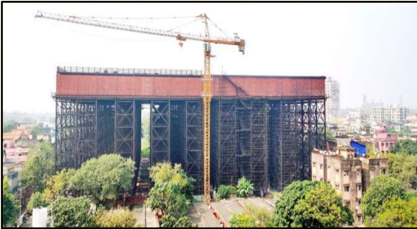
Renewing of 9.0 Mg Capacity Century Old Overhead Balancing Steel Reservoir (Tallah Tank) Under AMRUT for Kolkata Municipal Corporation (KMC)
