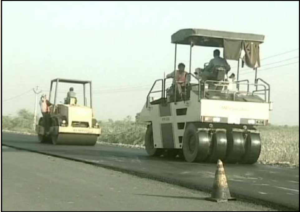
Strengthening and Paving of shoulders : Dholka to Bagodara (Km. 0.000 to Km. 23.000) and Wataman to Pipri (Km. 69.600 to Km. 94.000) for Government of Gujarat
