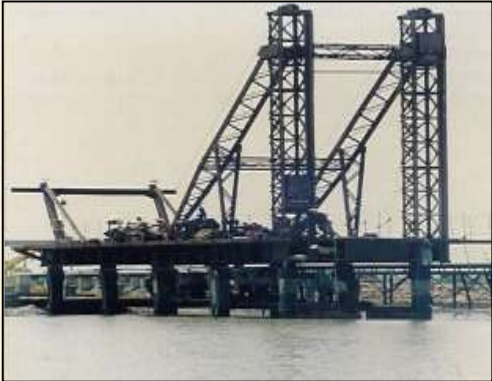
Pipeline Trestle Work for Construction of Jetty at Kakinada Coastal Installation for BPCL
