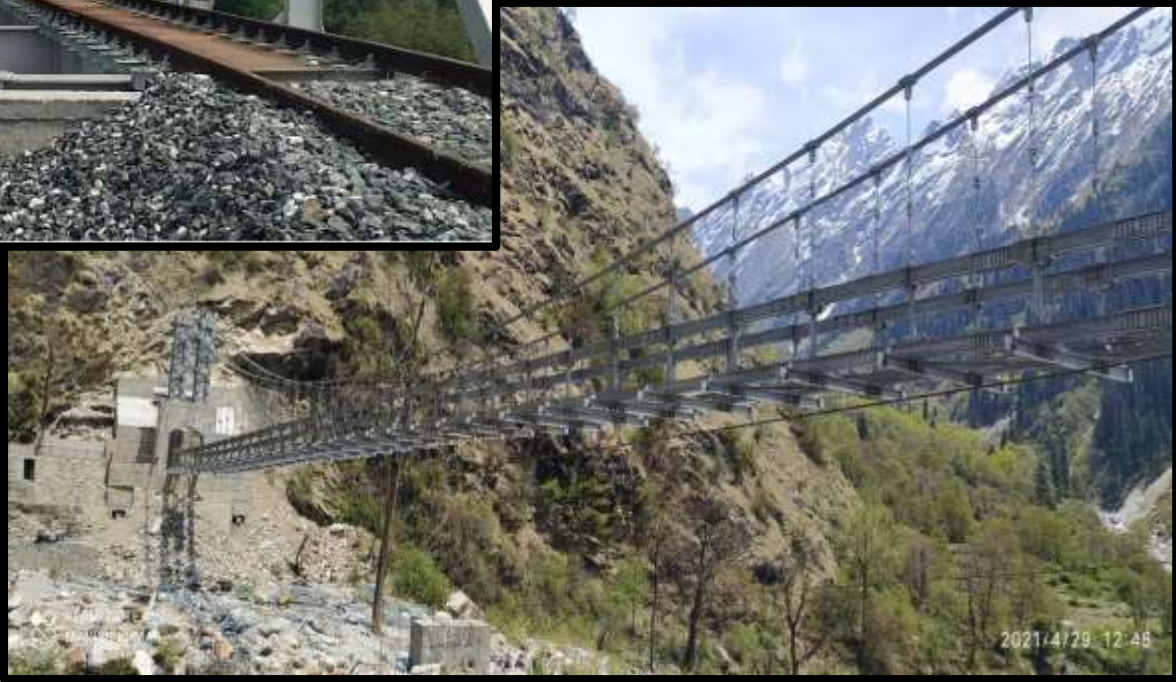
135 Mtr span Suspension Pedestrian Steel Bridge on Govindghat to Ghangharia Road at KM 10 in Chamoli District for PWD, Uttarakhand
