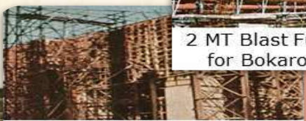
Civil Works for 3 X 200 MW Thermal Power Station at Obra for U.P.S.E.B
