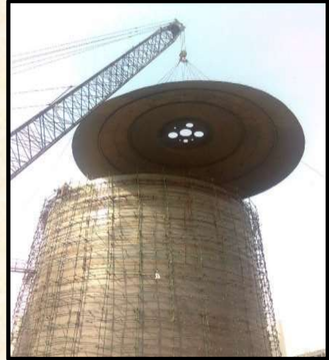
Double Walled Cryogenic Storage Tanks at IOCL Panipat Refinery
