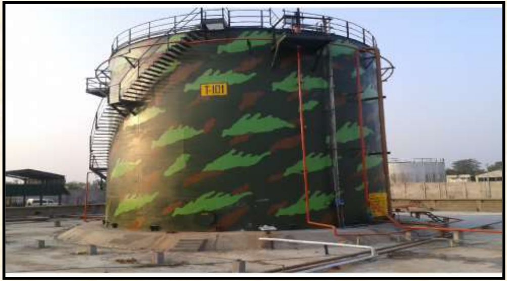
Turnkey Execution of Crude Oil Storage Tanks Fixed Roof Type at Mehsana Crude Tank Farm of ONGC
